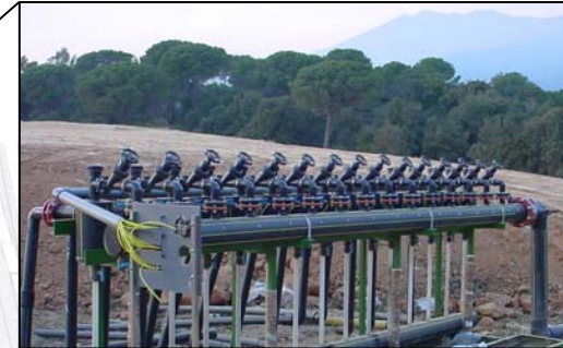
Regulation and control station
