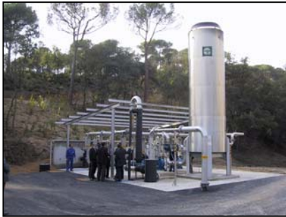
Flare and combustion plant
